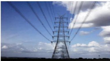
During April this year, peak power demand met or the highest supply in a day touched the highest level of 182.55 GW and recorded a growth of nearly 38 per cent over 132.73 GW recorded in the same month in 2020.
